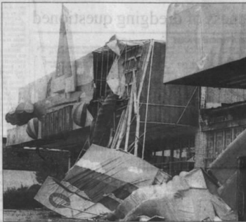
Buildings show damage by winds from Hurricane Bonnie Wednesday at North Myrtle Beach, S.C. Taking one of the city's busiest storm routes, Hurricane Bonnie blew into the Carolinas with 115 mph winds.
