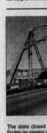
The state closed the Michigan Street Bridge to vehicles Friday so repairs could be made.
